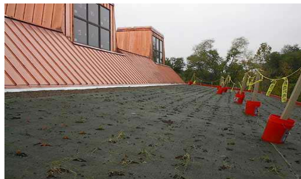
Finished rows of plants are set to grow on the northwest side of the roof.
