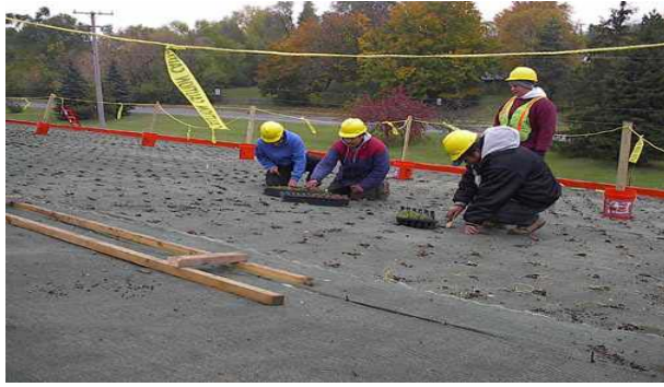
Workers plant various varieties of sedum on the northeast side of the roof on October 28, 2003. Plants are spaced 12 inches on center to cover the 13,000-square-foot roof.
